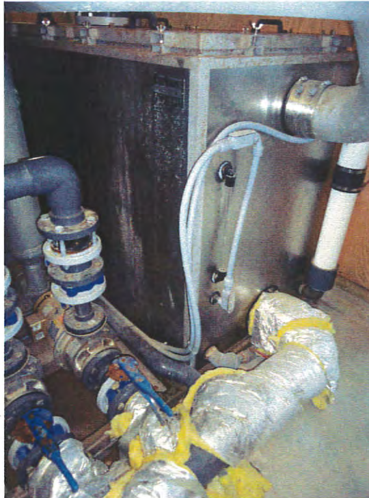
Photo 3; Lowry Aeration Equipment
